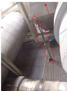
Picture 2 - Boiler ash injection pipe
